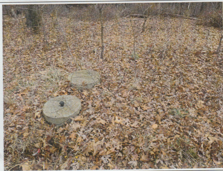
Photo #: 2 Taken By: Grant Bicker Facility: Eagle Bay Location: 28451 Northwood Drive, Lincoln, MO Description: The dump station located east of the swimming pool. Date Taken: December 16, 2022 Program: Water Pollution Control Unit
