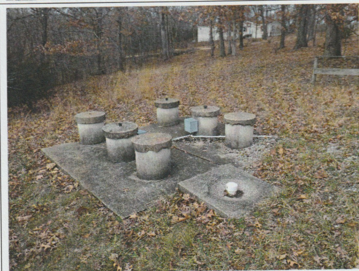
Photo #: 3 Taken By: Grant Bicker Facility: Eagle Bay Location: 28451 Northwood Drive, Lincoln, MO Description: The dump station near the shower house. Date Taken: December 16, 2022 Program: Water Pollution Control Unit
